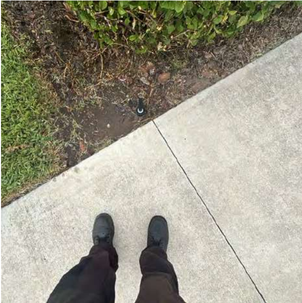
Zone #3 (Clogged Nozzle) - 06-09-26 8:35 am CDT
