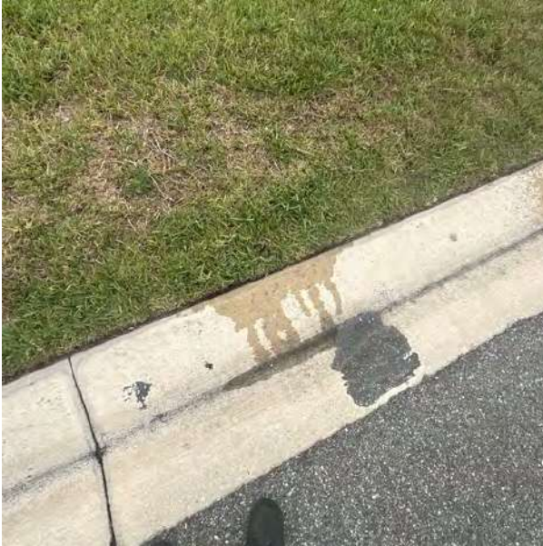
Zone #40 (Clogged Nozzle) - 06-09-26 10:39 am CDT
